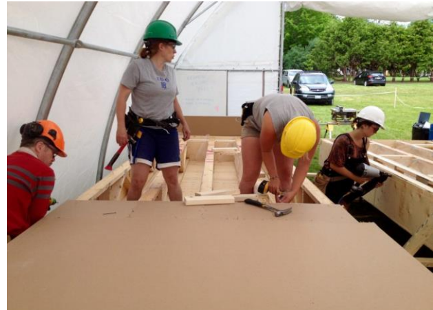
ReWall EssentialBoard, made from 100% recycled food and beverage cartons, was used in the Zero House green building project. Photo Credit: Zero House
